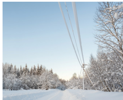
3. Winter storms can cause major damage to power lines and other electricity delivery infrastructure. Ice can form on power lines, causing them to sag or even break. Such events have caused major power outages in recent years. Courtesy: koldunova / Envato Elements
