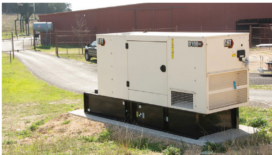
3. A Cat D100 GC diesel generator set provides backup power for a wildlife ranch. Courtesy: Cat Electric Power
