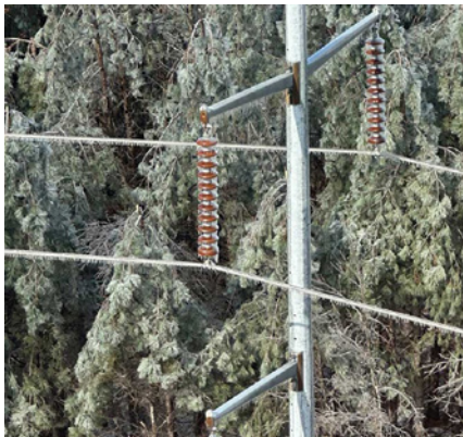
3. Ice accumulation on Tennessee Valley Authority (TVA) transmission line conductors during Winter Storm Fern. TVA transmission lines are designed to withstand 0.25 to 1.6 inches of ice depending on conditions, and design tension is limited to account for extreme cold and ice loading. TVA reported that no structures or conductors failed solely due to ice and wind during the storm. Failures occurred only where falling trees added weight to lines. Source: Tennessee Valley Authority
