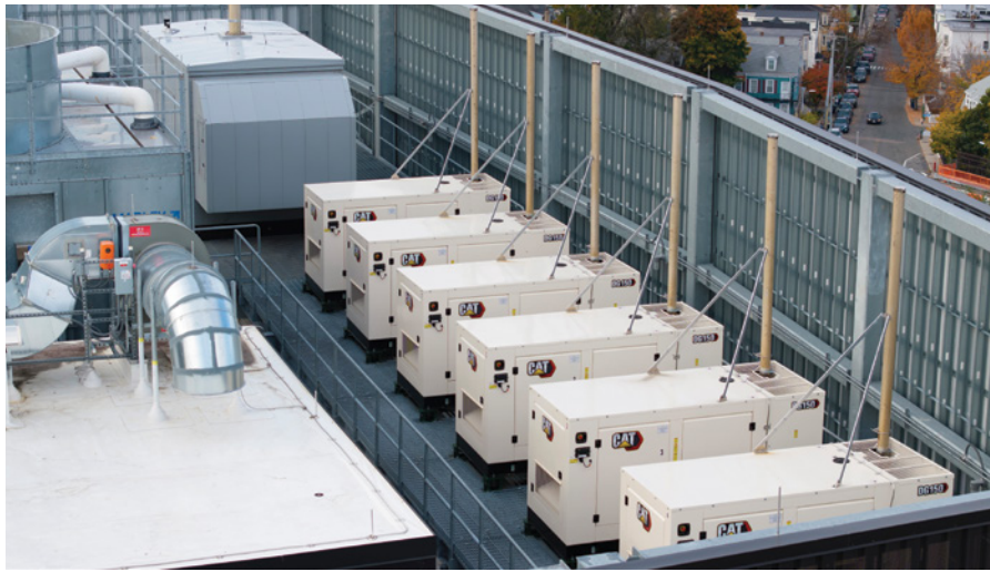
1. Six Cat DG150 gas generators provide reliable backup power for a state-of-the-art life sciences hub. Courtesy: Cat Electric Power
