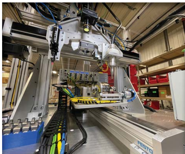
A closeup view of the Y axis, center, and the Z and X axes. On the Z axis from left to right are the Nordson adhesive applicator, Banner vision system and plasma gas applicator. The pick-and-place guided actuator is mounted behind the plasma applicator and is not easily distinguished. A box of die-cast housings is visible on the lower left.
