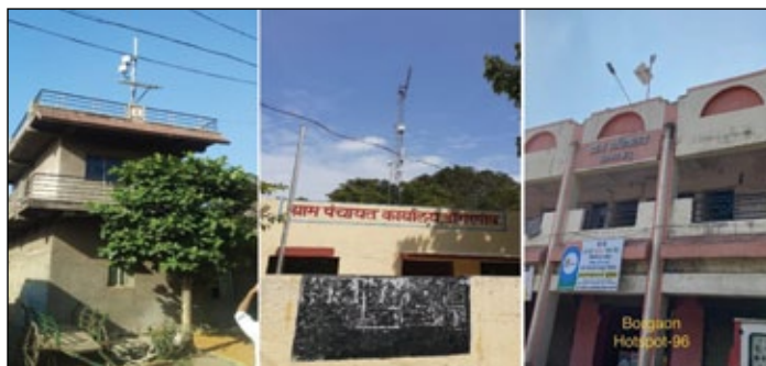
C-DOT Wi-Fi Installation at Akola Maharashtra
